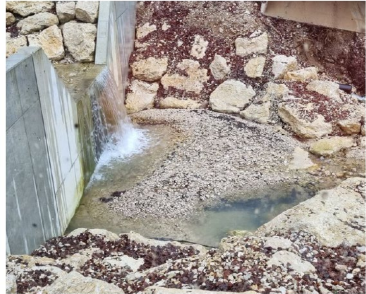
Figure 13. Picture of the sediment accumulating in the dissipation pool after the first sill in the upstream basin, taken after the winter 2023-2024. Courtesy of ATB SA.
