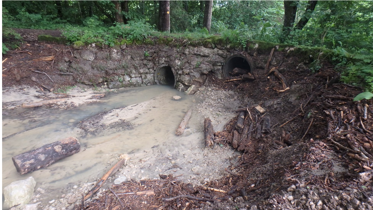
Culverts after the flood of 2018
